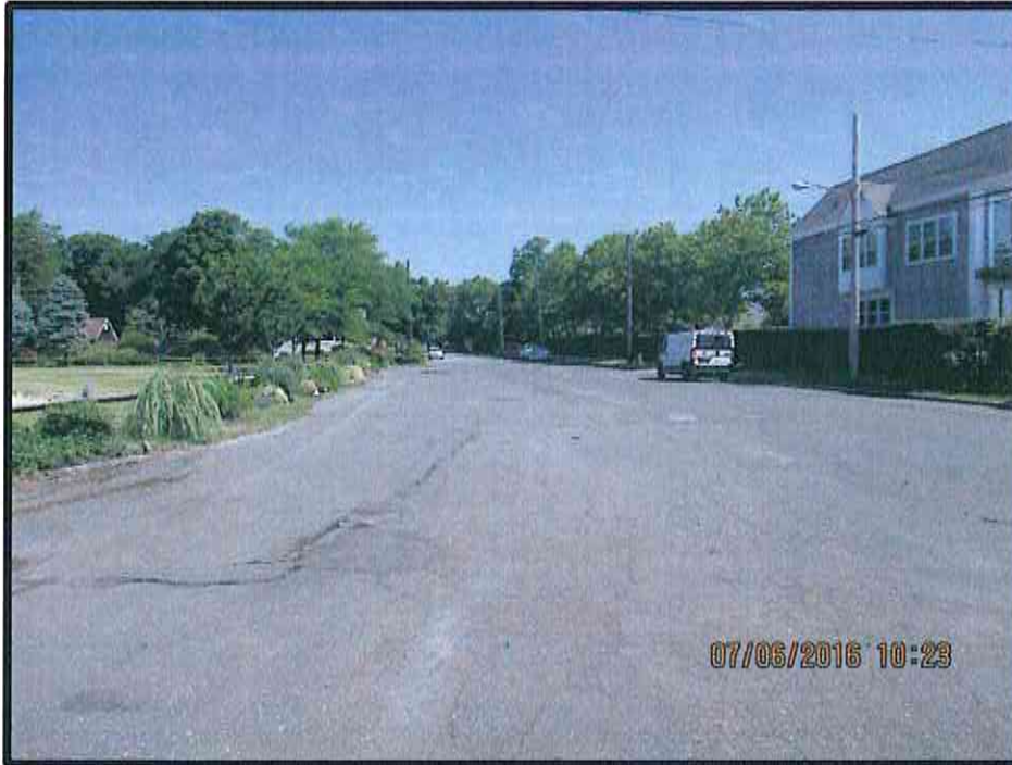
Photo 39 – View looking north on Fifth Street; adjacent to Village of Greenport park.
