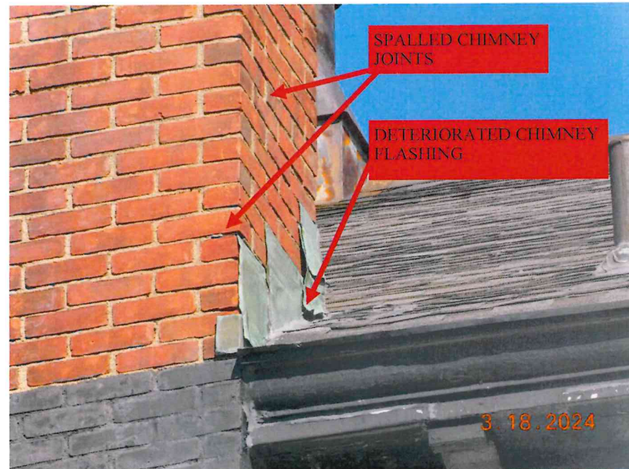
PHOTO NO. 08 MAIN ROOF CHIMNEY DEFICIENCIES
