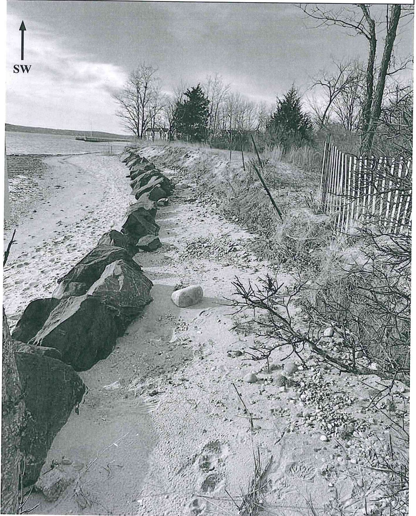
Figure 2. A photograph of the erosion damage to the coastal dune illustrating how the boulder toe acts to channelize the waves along the dune face.
